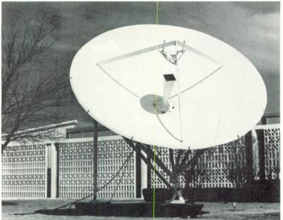
Ten-meter earth terminal antenna for both uplink and downlink is the type put into use on January 1 by Enterprise Radio at their Connecticut headquarters
